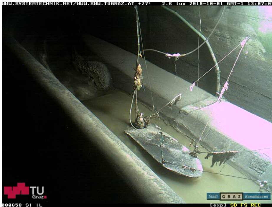
Figure 2. UV/VIS s::can® spectrometer installed in swimming pontoon in a combined sewer overflow structure in Graz. The sensor is always located in the top water layer and subsequently measures the water quality, which is discharged at the overflow weir during storm flow conditions. Measured parameters are COD_{eq} , T(D)OC_{eq} , TSS and NO_3-N_{eq} . Picture shows probe after storm-water event. © G. Gruber, TU Graz
